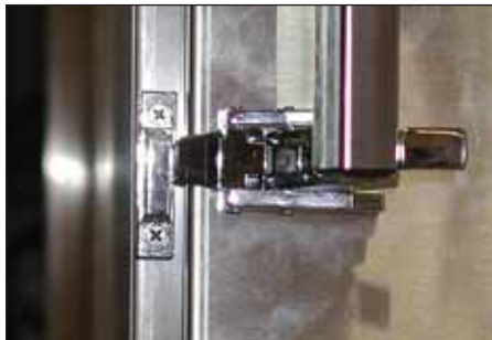
Door Latch Too High
